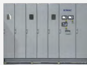
Motor inverter panel
